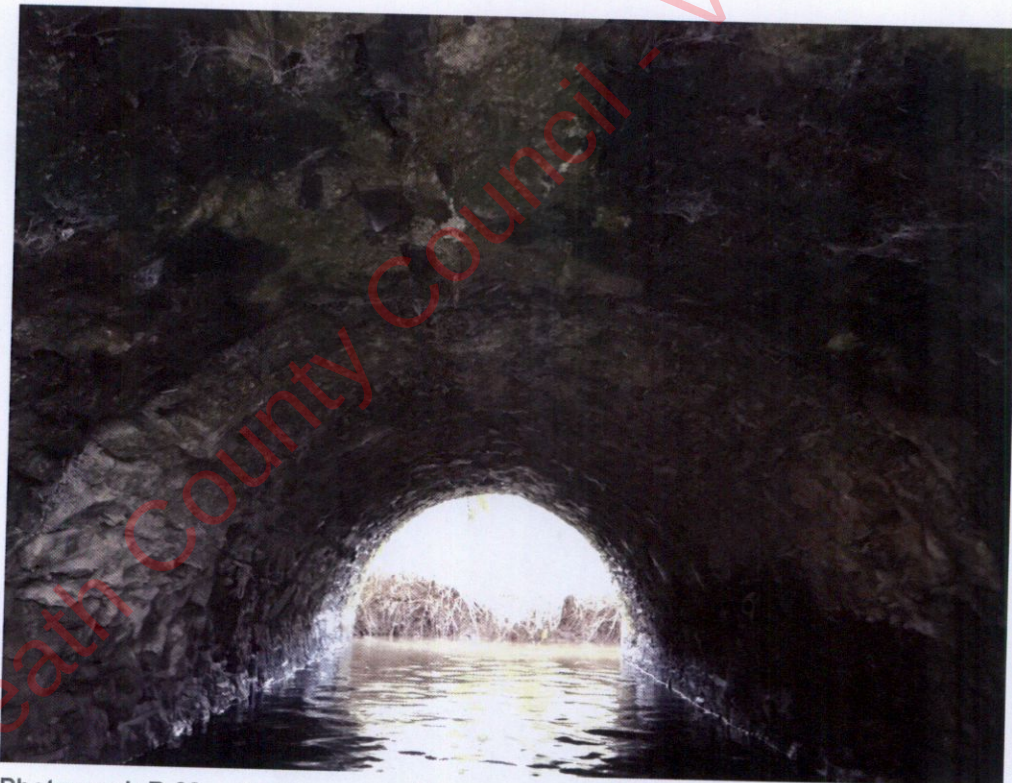
Photograph B-28 – Arch barrel 6 with water ingress and minor pointing loss evident
