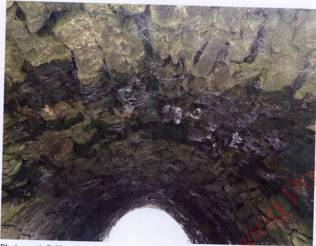
Photograph B-23 – Arch barrel 1 with pointing loss and water ingress evident
