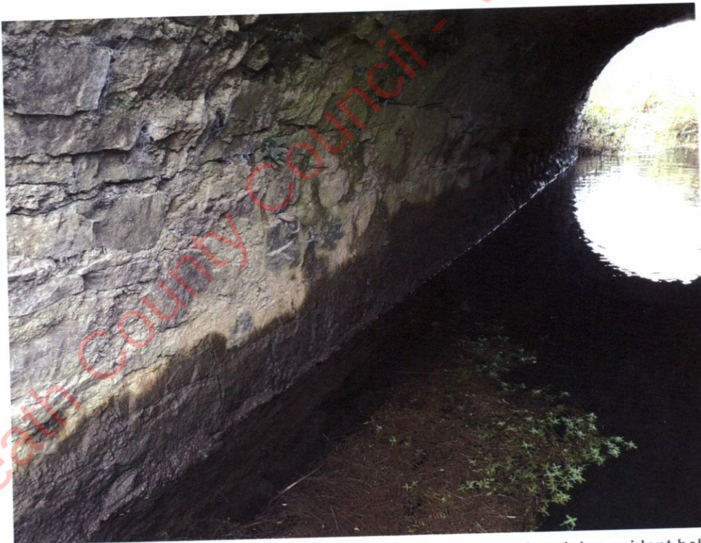
Photograph B-12 – North abutment with pointing loss and undermining evident below waterline
