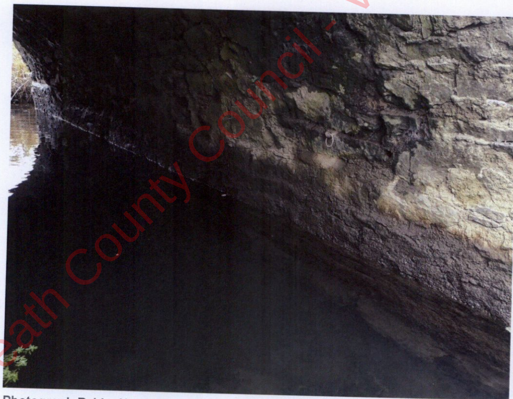
Photograph B-14 – North face of pier 1 with undermining evident
