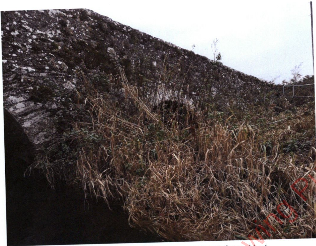
Photograph B-7 – NE embankment with overgrown vegetation evident
