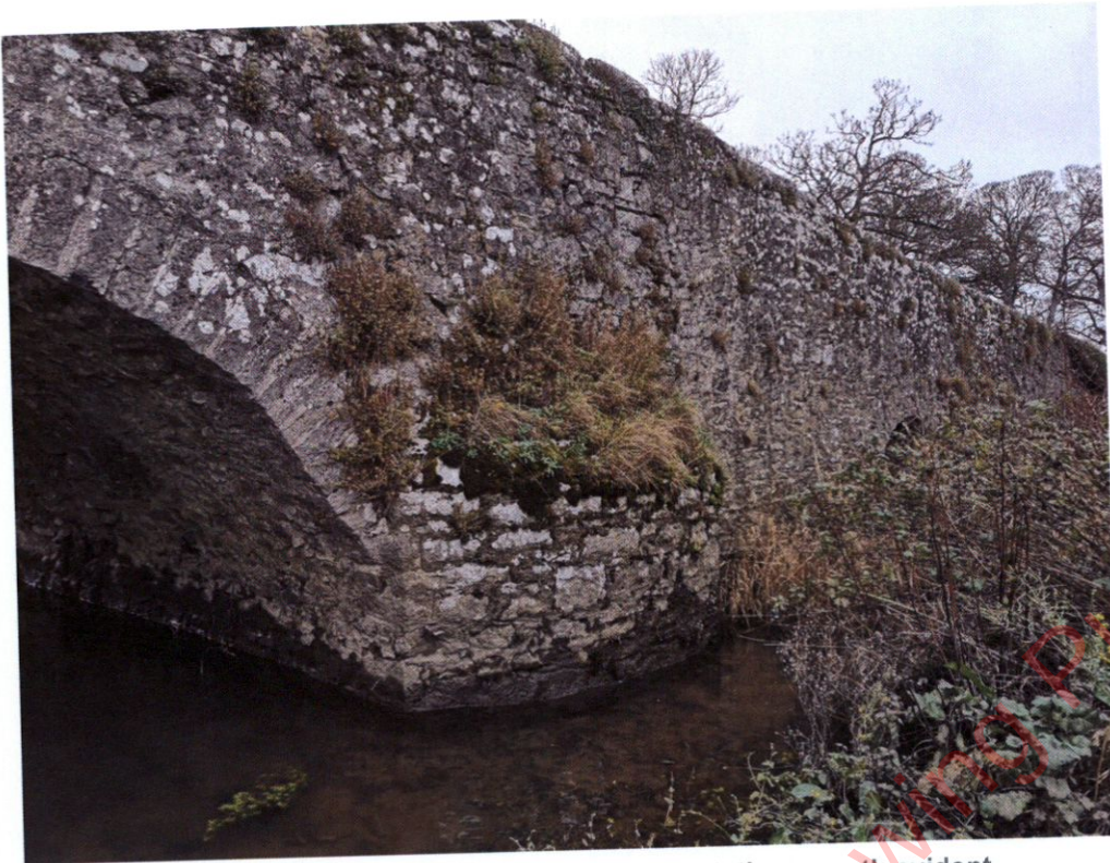
Photograph B-19 – West cutwater of pier 4 with vegetation growth evident
