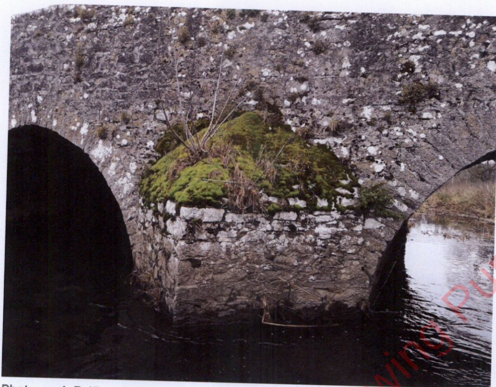
Photograph B-17 – West cutwater of pier 3 with vegetation growth evident
