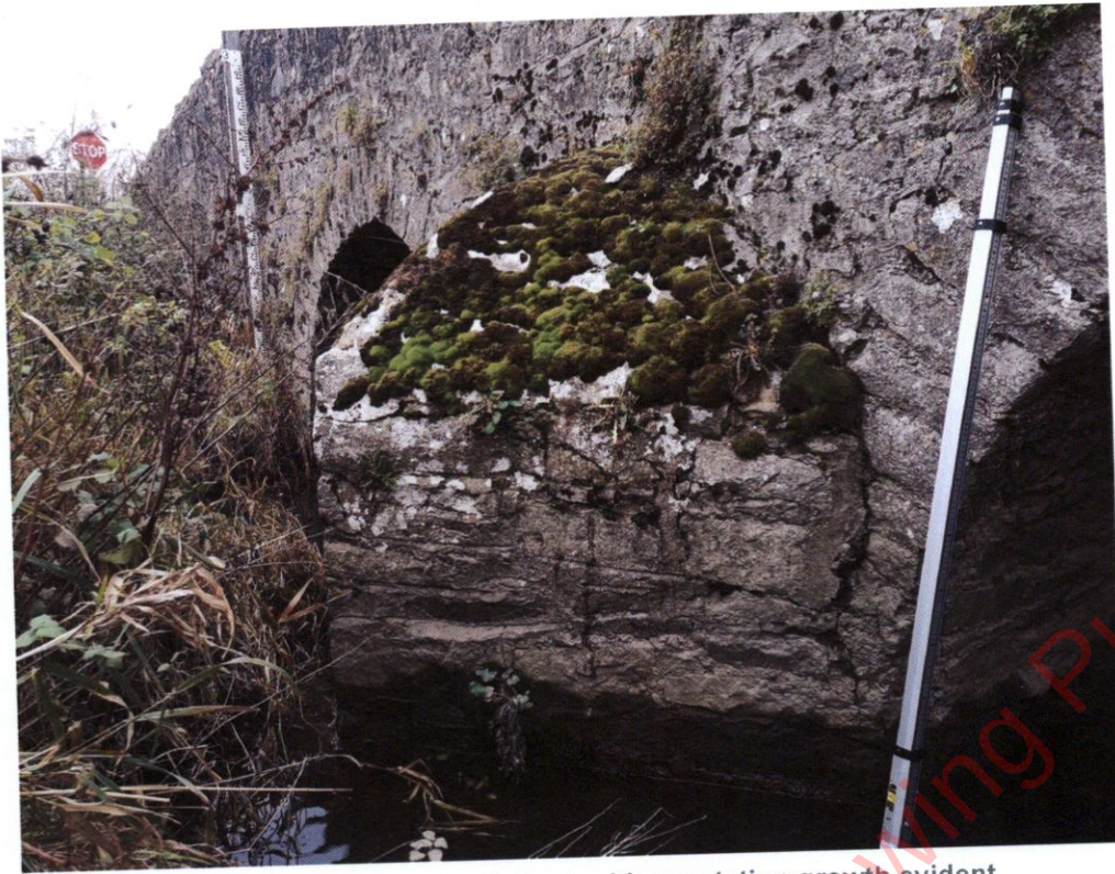
Photograph B-15 – West cutwater of pier 1 with vegetation growth evident
