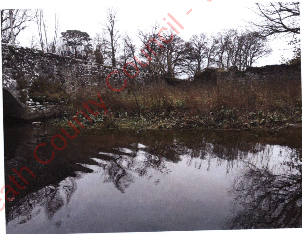
Photograph B-8 – SW embankment with overgrown vegetation evident
