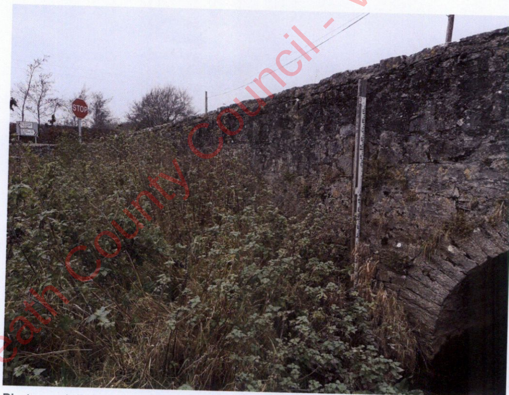
Photograph B-6 – NW embankment with overgrown vegetation evident
