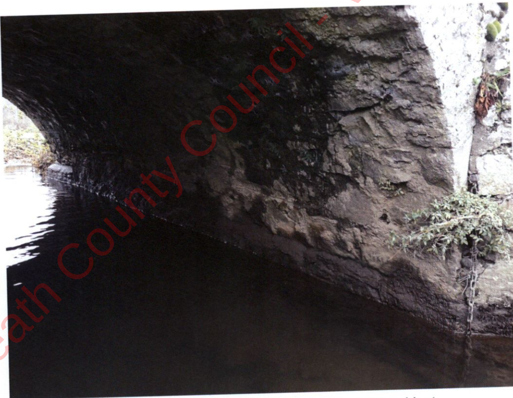
Photograph B-16 – North face of pier 2 with vegetation growth evident
